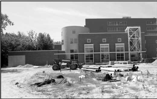
Current construction on Morris deals with the atrium of the new north entrance, the entry plaza, and the water feature.
